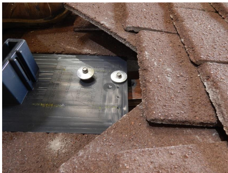
Figure 5 Image to indicate the fixing of the brackets with the clay tiles.
