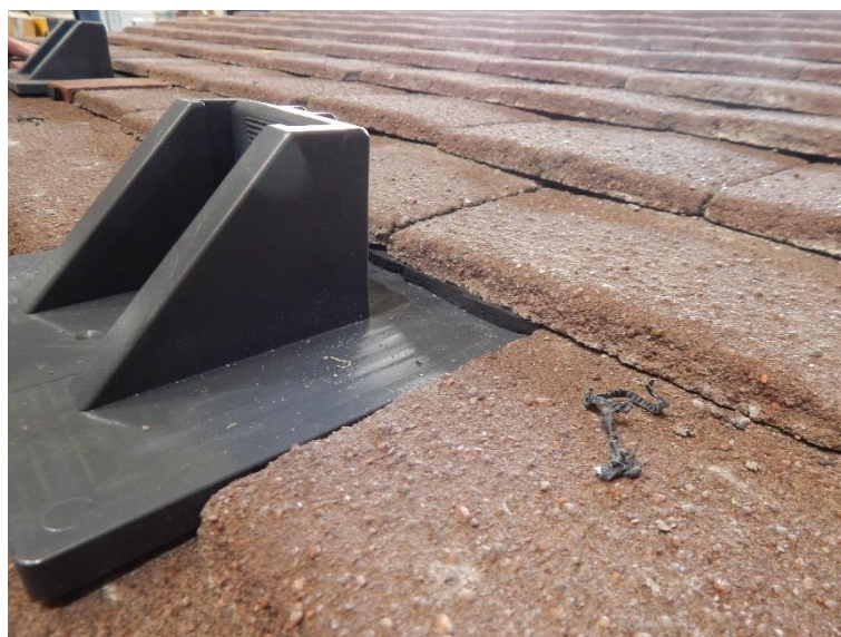
Figure 9 Image to highlight the gap created by the installation of the PV bracket with plain tiles and the EDPM foam used to seal the gap.
