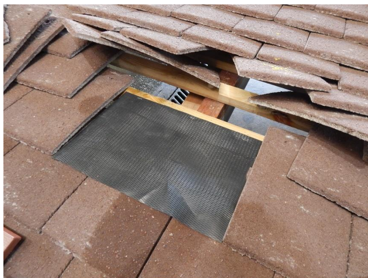
Figure 7 Inclusion of a standard damp proof course layer ensured weathertightness was maintained.
