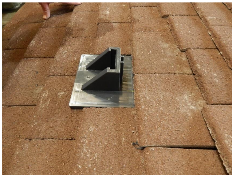
Figure 6 Image to highlight the test set up for the brackets with clay tiles.
